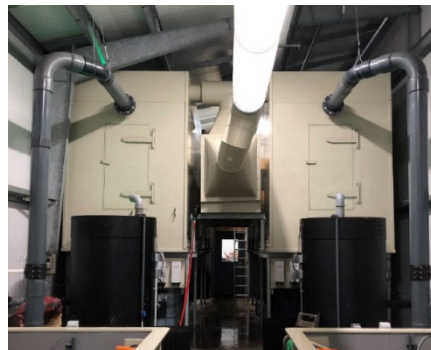
HEAT RECOVERY VENTILATOR (CENTER) WITH SUPPLY AIR DUCTING AND OXYGENATORS (BLACK TANKS) ON EITHER SIDE.
