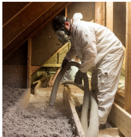
THIS PHOTO, TAKEN FROM A RGGI FUNDED RESIDENTIAL INSULATION PROJECT, REPRESENTS THE KIND OF ATTIC, CRAWL SPACE, AND EXTERIOR WALL INSULATION WORK THAT IS SUPPORTED BY HPWES AND THAT WAS IMPLEMENTED FOR THE AFOREMENTIONED
