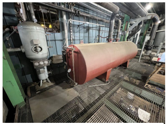
Flash tank with shell and tube heat exchanger (L) and condensate reservoir (R)
